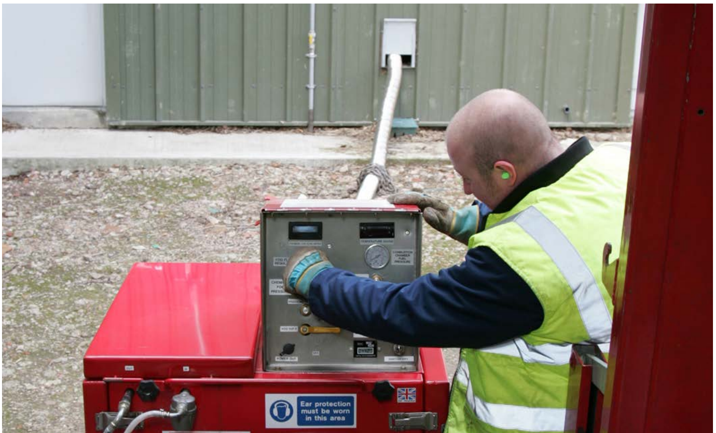
Figure 29. Hot-fog application of CIPC
