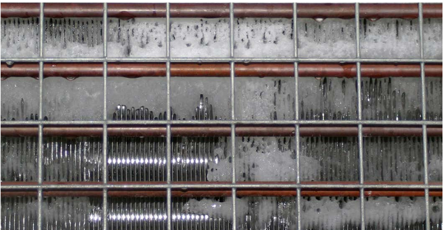
Figure 21. Ice must be regularly cleared from cooling coils
