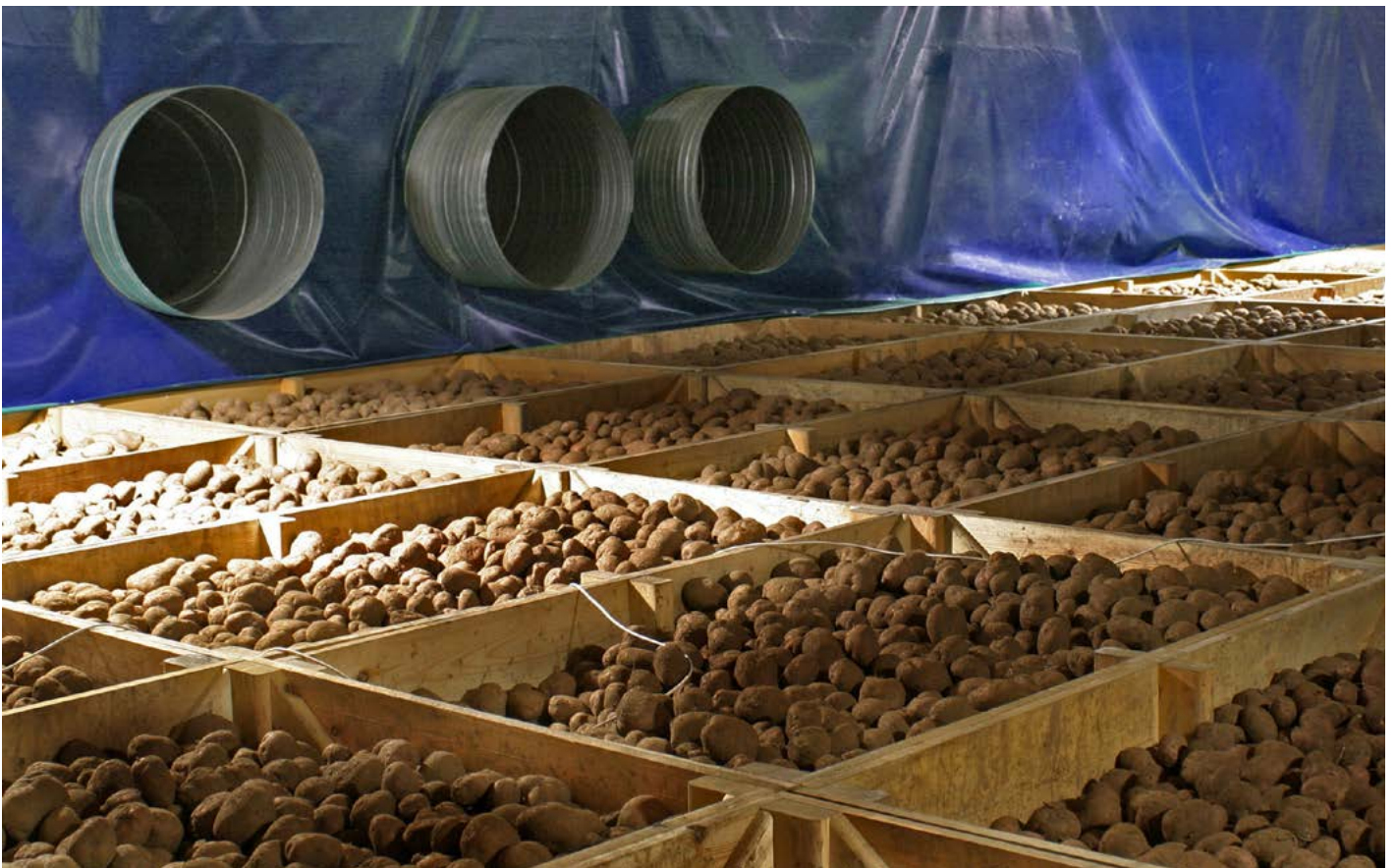
Figure 11. An air separator curtain boosts ventilation efficiency significantly by preventing short circuiting
